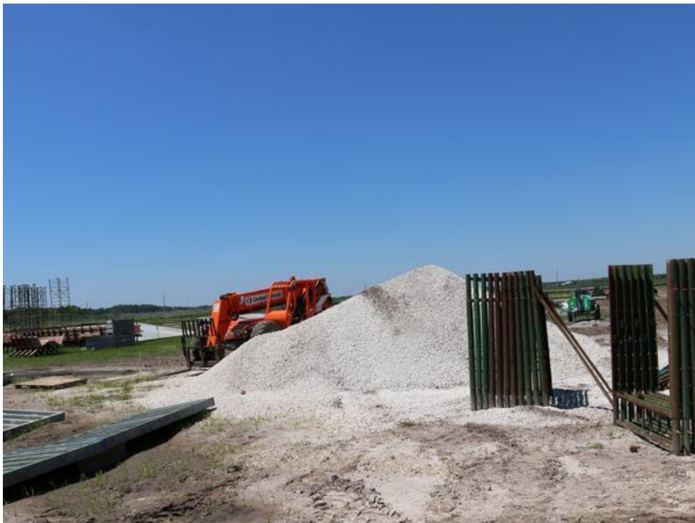
Hundreds of tons of rock is used to prevent slips and falls from workers and to help machinery move uphill. Matthew Richardson
