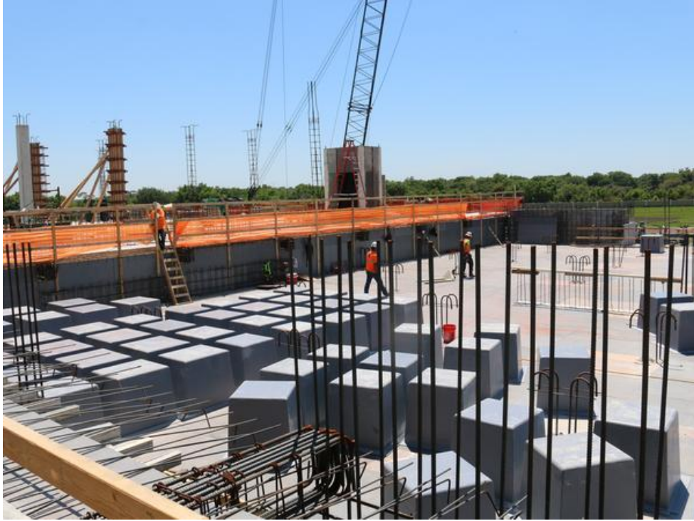
The waffle design is what helps better circulate clean airflow to the clean rooms. Matthew Richardson
