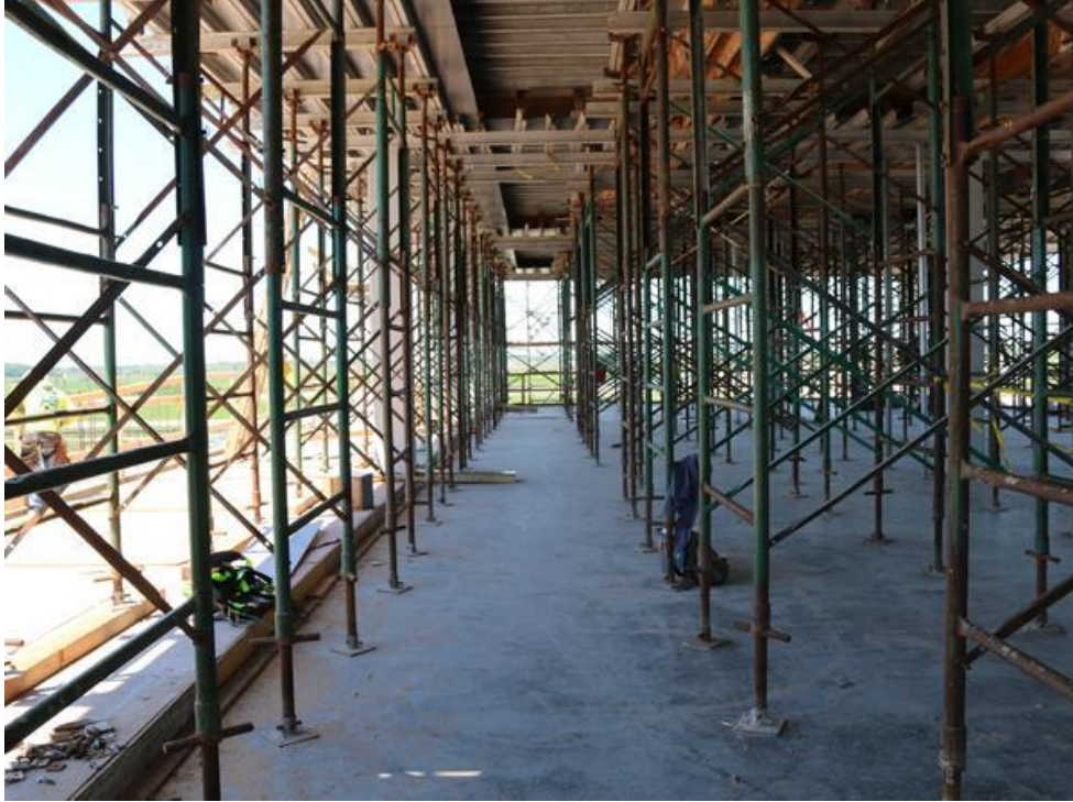
Rows and rows of steel pipes. This is the second level of the center. Matthew Richardson
