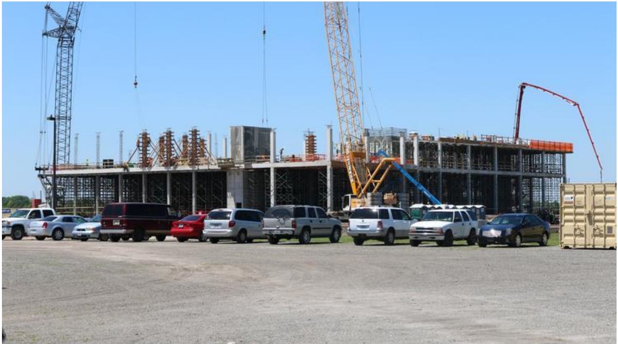
Here's a look at the back of the FAMRC. Vertical work has been taking place for 34 days. Matthew Richardson
