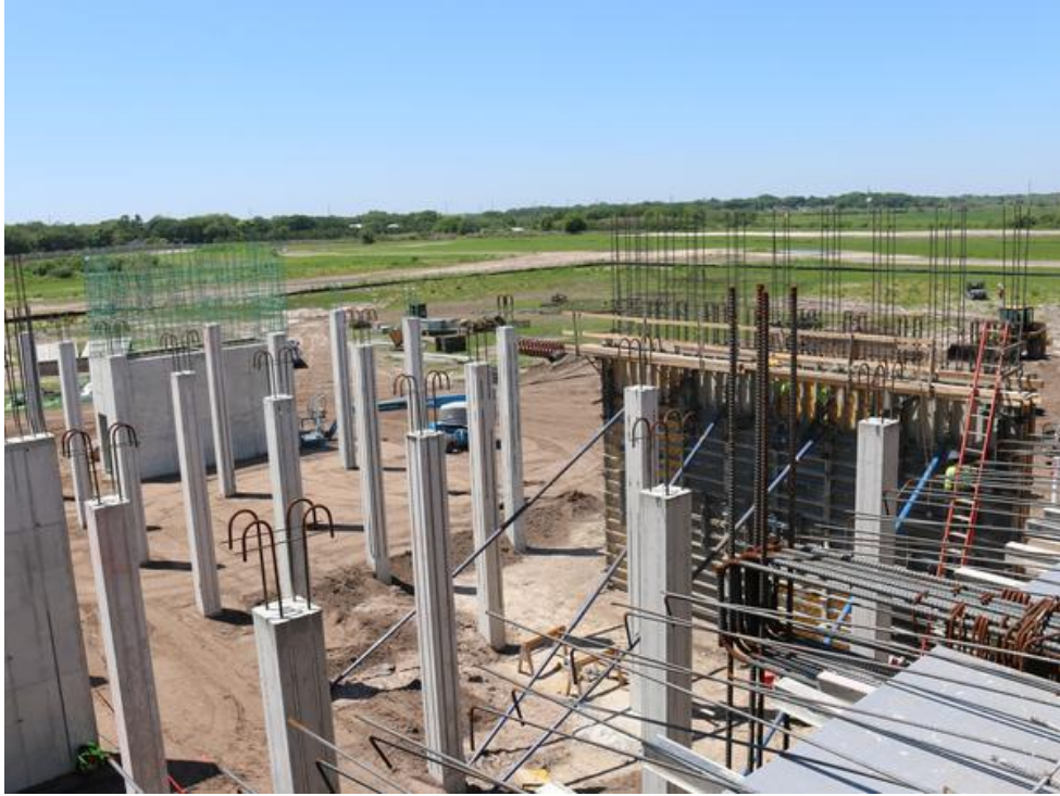
See all the concrete pillars? Those were formed using a casting method instead. Matthew Richardson
