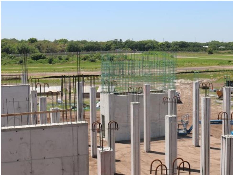
See the area with the green steel pipes? That is where the electromagnetic microscope will be held. Special attention is given to that area because that particular room has to be ultra stable to prevent shaking. Matthew Richardson
