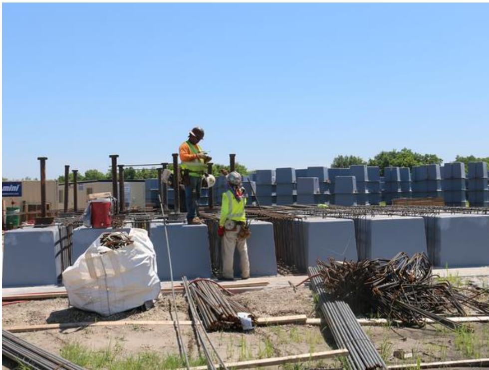
The waffle design is tied together using steel pipe before being lifted in the air. Matthew Richardson
