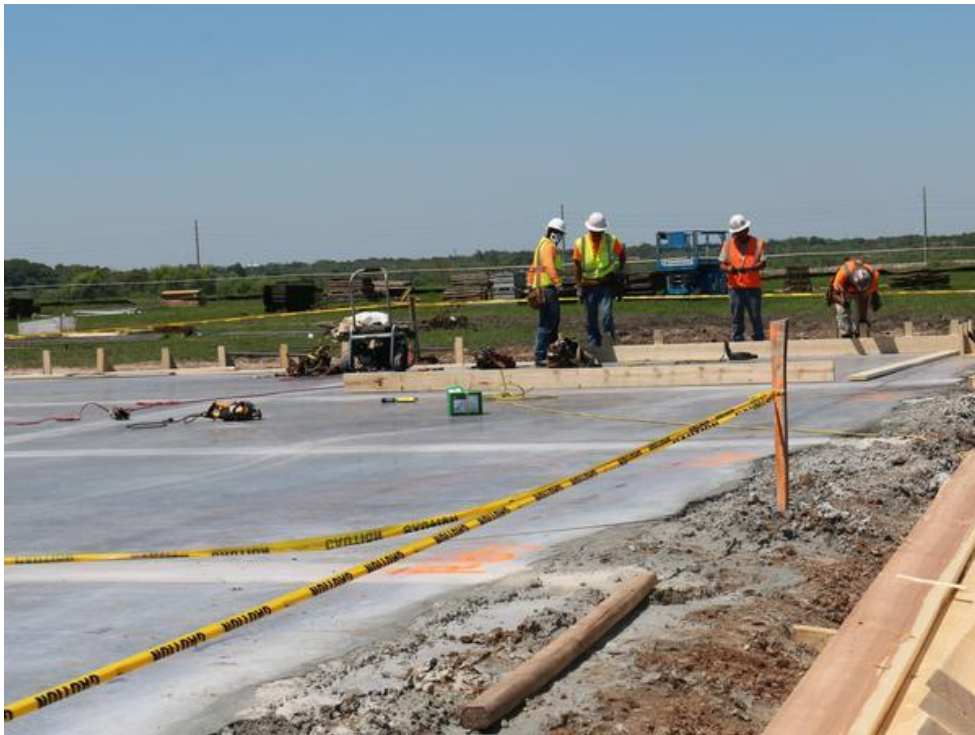
This is a different process than usual for buildings. This process is used for the FAMRC because of the need for tall, solid concrete walls. Matthew Richardson
