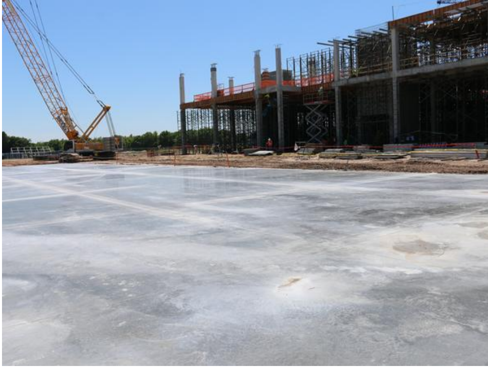
Here's the concrete casting bed. Cement is laid to dry and later broken up to create the walls for the building. Matthew Richardson
