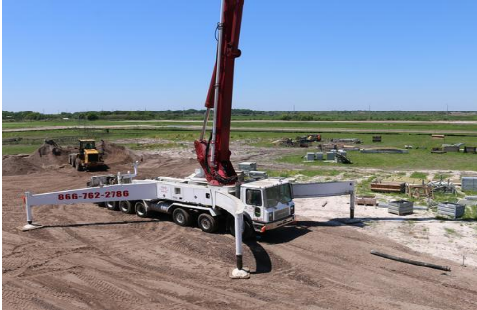
This vehicle funnels cement into a casting tower to form large concrete beams. Matthew Richardson
